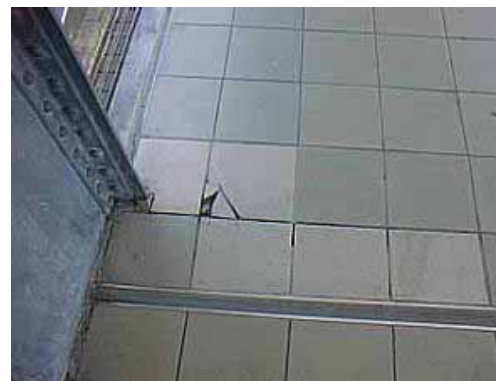
Ramped walkway surface 'before'.
