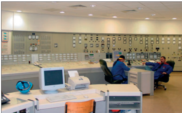
The modified control room
